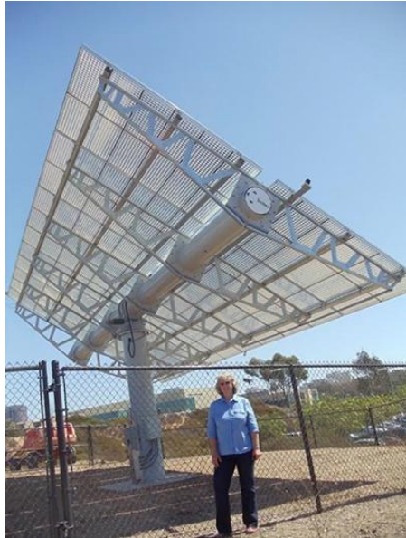
Figure 2. A CPV solar tracker installed on the UCSD campus.
